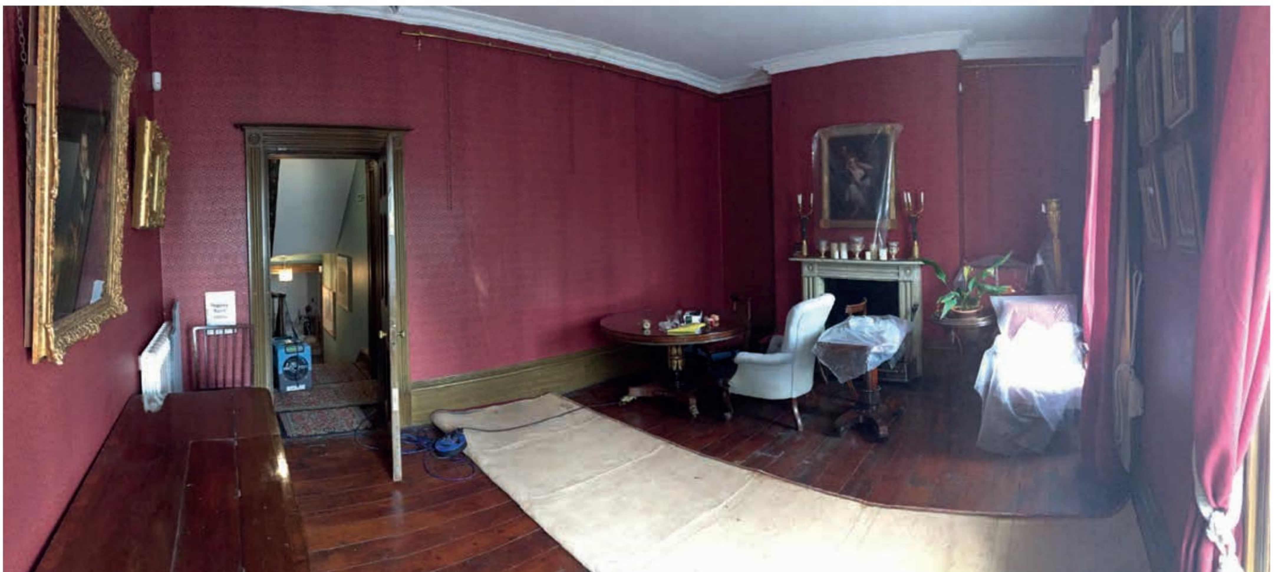
Flood damage in the Regency Sitting Room, Holst Birthplace Museum © Holst Birthplace Trust
